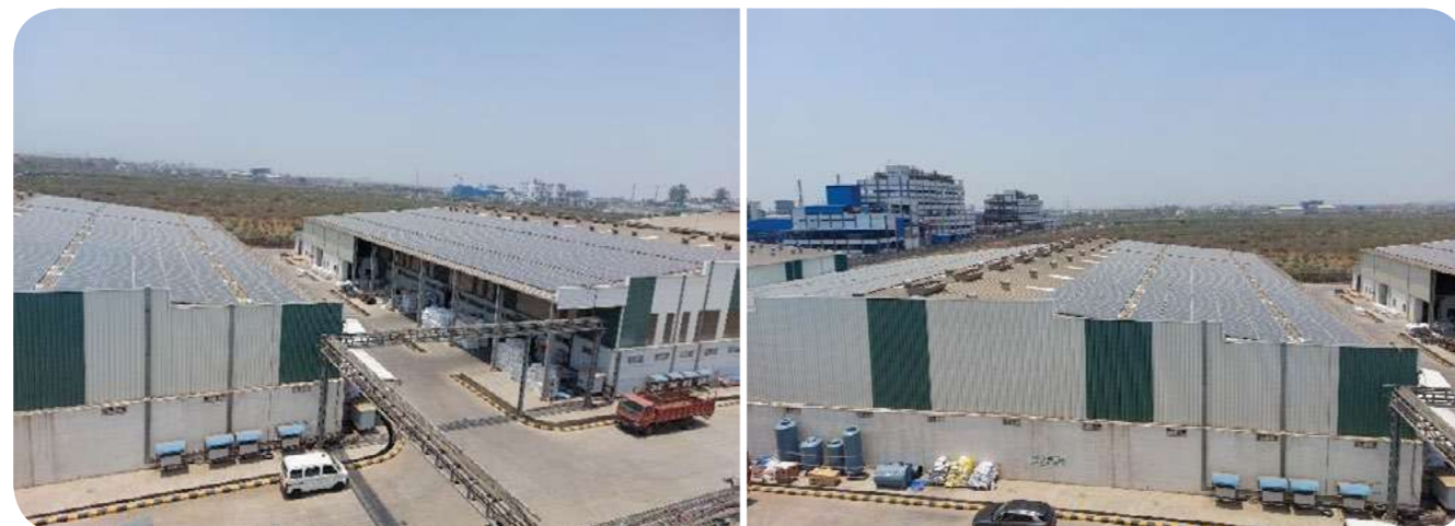
Solar Panels installed in Warehouse of Dahej plant which leads to reduced green house effects
