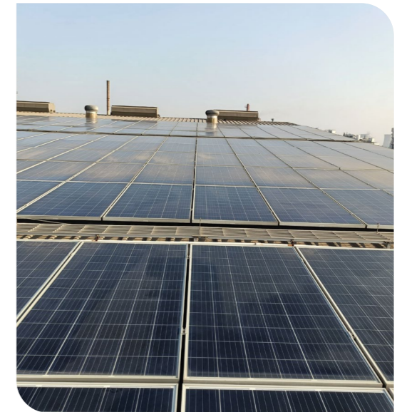
Solar Panels at Chopanki Plant
